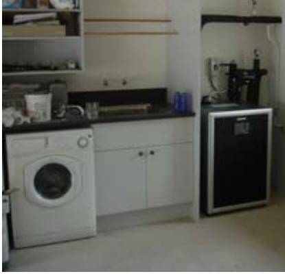
Typical utility room installation of a ground sourced heat pump
