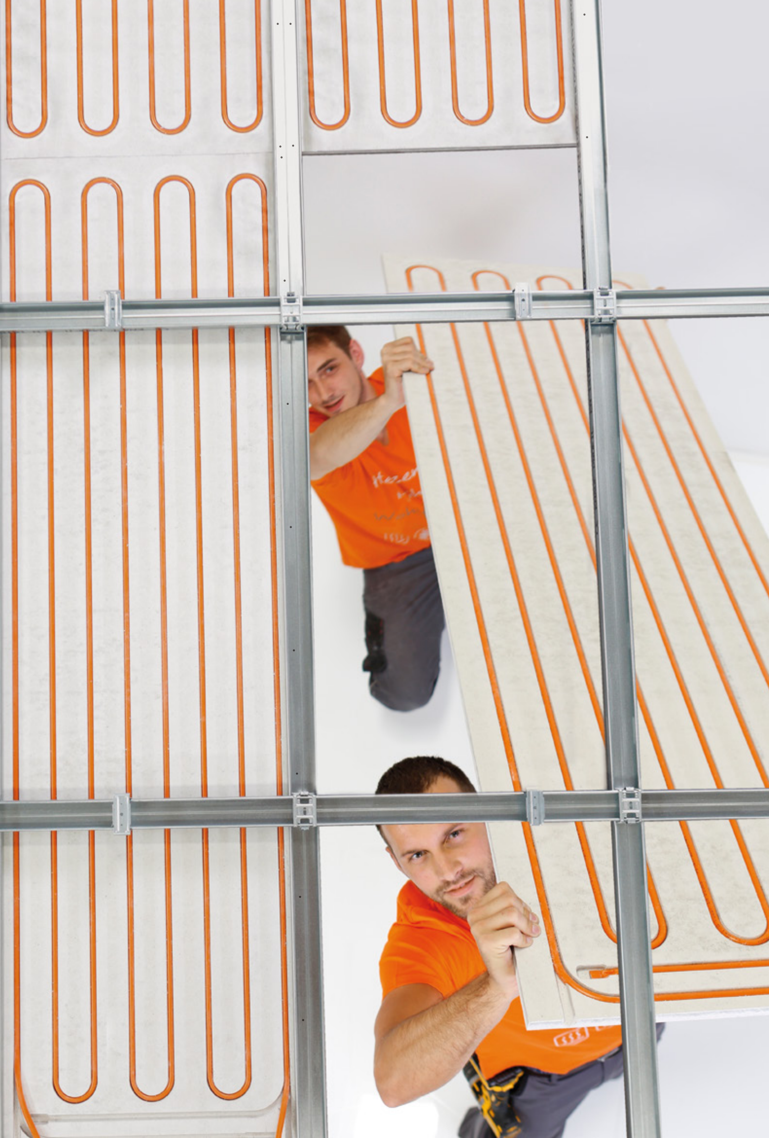
MODULAR CEILING COOLING | MODULAR CEILING HEATING
