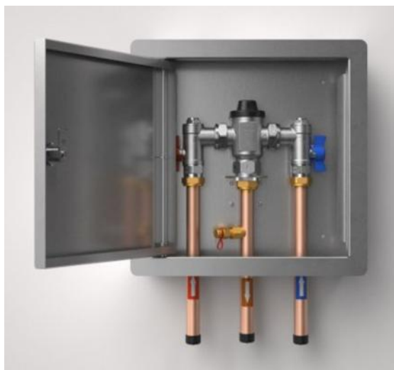
Figure 1: Mixing valve set in recessed hatch
