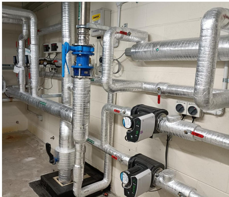
Figure 13: DHW plant insulation of the highest standard
